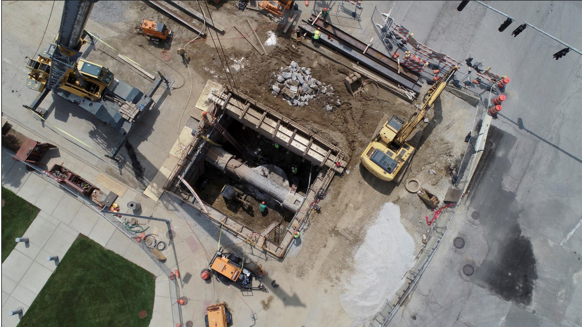
Jackson / Superior Drop Shaft Construction Photo Taken by David Patch, Photographer for The Toledo Blade
