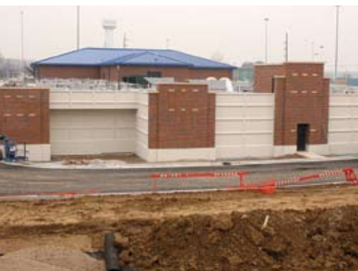
The new Wet Weather Facility at the Bayview Wastewater Plant was completed in 2006 and is now operational.
