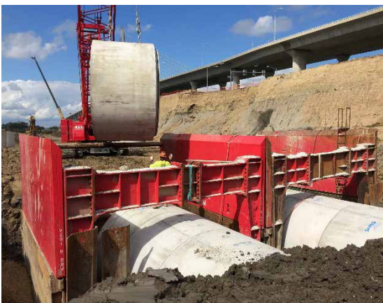
A crane maneuvers a section of precast pipe into place during construction of the Dearborn CSO Storage Pipeline.
